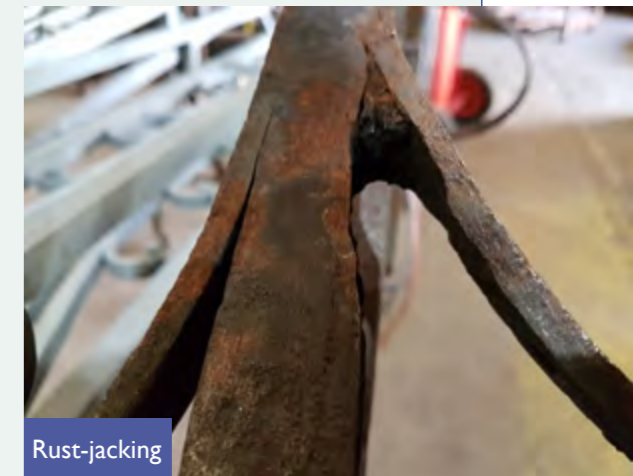
Blistering, pitting and rust-jacking
