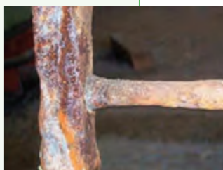
Top: Wrought iron stile and rail: - 1858 - material sections still intact
